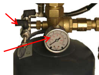
Water supply manometer
